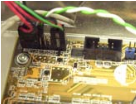
2.5.Connect LED's and Front Panel Leads to MB -Power SW: Connect to MB "PWR" -Power LED: Connect to MB "PLED" -HDD LED: Connect to MB HDD/IDE LED connector -Reset SW: Connect to MB "RSW" -Speaker: Connect to MB 4-pin connector
